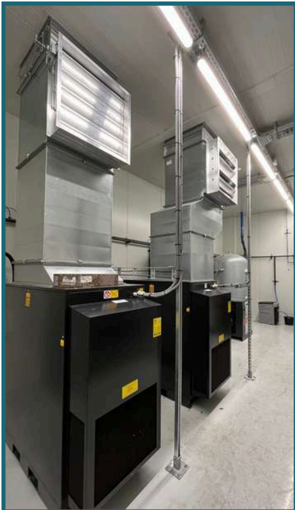
Two frequency-controlled compressors, Warehousing Botlek
